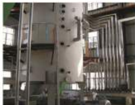
浸出车间蒸发器 Desolventizer-Boiler of Extraction Workshop
