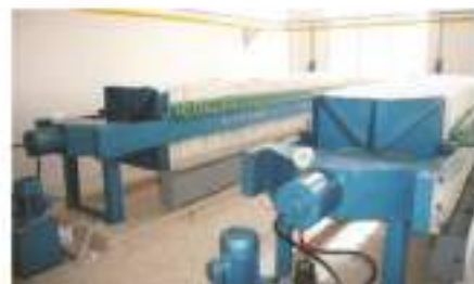
板框过滤工序 Plate-frame Filter Process
