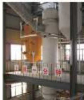
浸出车间蒸发系统 Evaporation System of Extraction Workshop
