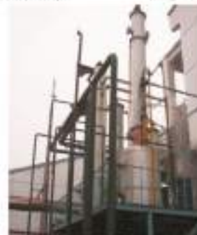
浸出设备尾气回收 Solvent Recovery From Vent Gas
