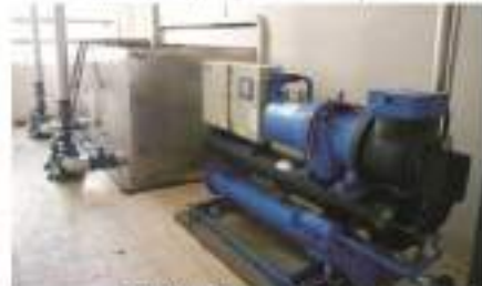
冷冻系统 Refrigeration System
