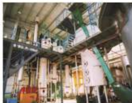
浸出车间蒸发系统 Evaporation System of Extraction Workshop
